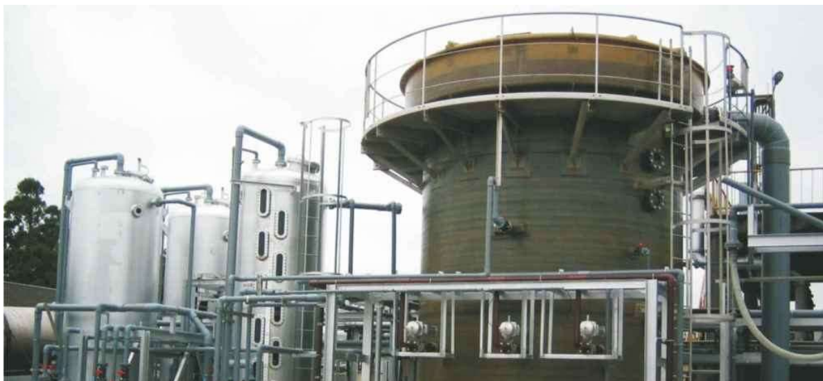
Figure 6 A view of a tank (on the right-hand side) in which the ion-exchange resin is held at this site in Japan.
